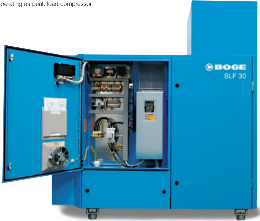
The frequency convertor with its built in control is integrated neatly into the existing electrical cabinet.
